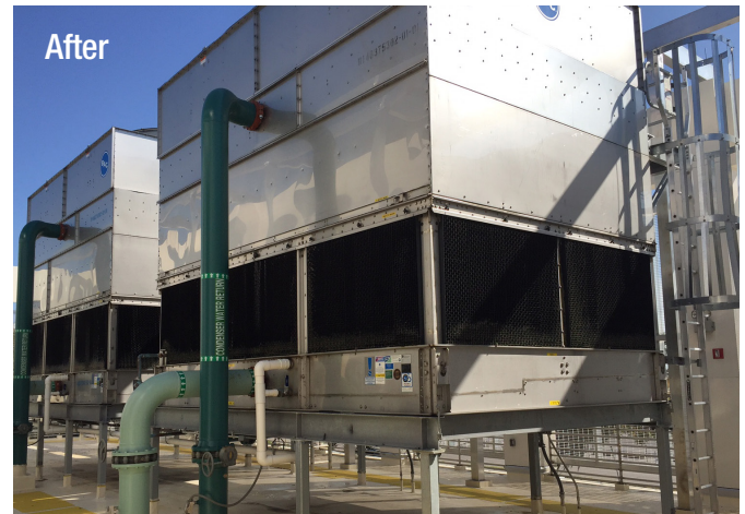
Old, failing chillers were replaced with new, high-efficiency chillers on the roof of the newly constructed District Cooling Plant.
