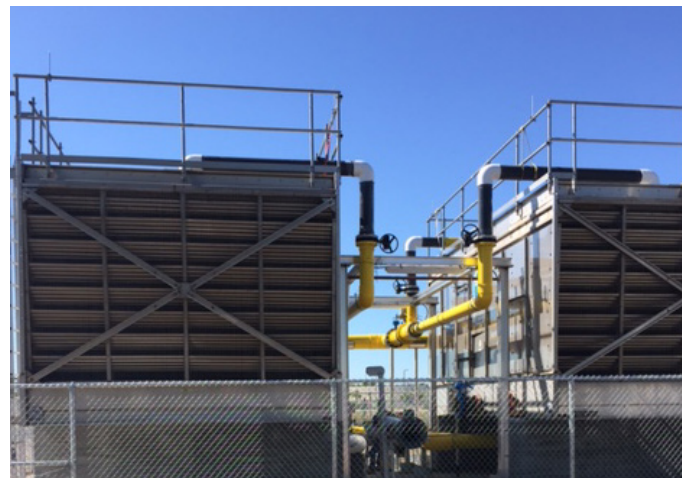
The combined use Chiller Plant replaced old, failing chillers and takes advantage of utility Time-of-Use rates
